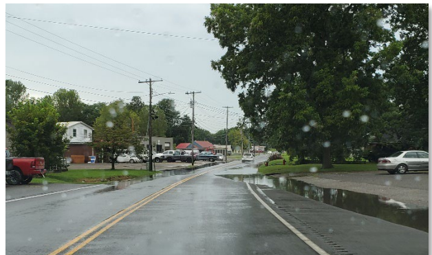
Drainage issues along KY 58
